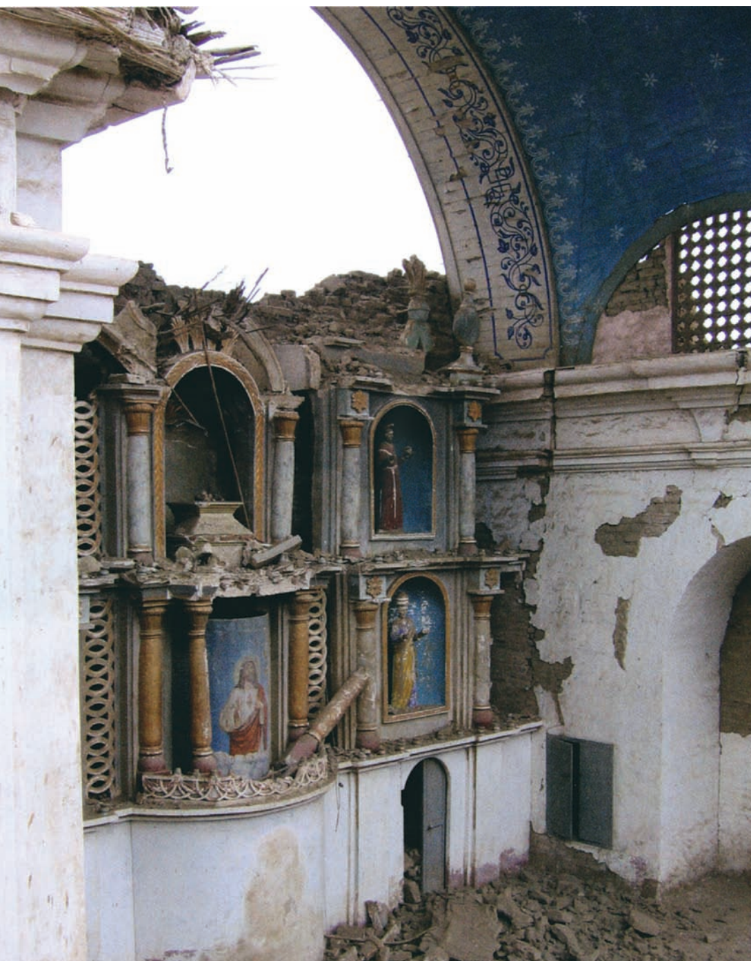
The altar of the church of San Pedro in Coayllo, after the earthquake of August 2007 (Photo: Rommel Angeles Falcon)
