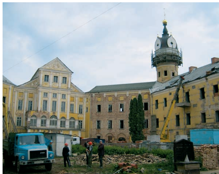
Hrodna, Old Castle, inadequate renovation work (Photo: A. Milinkevich)
