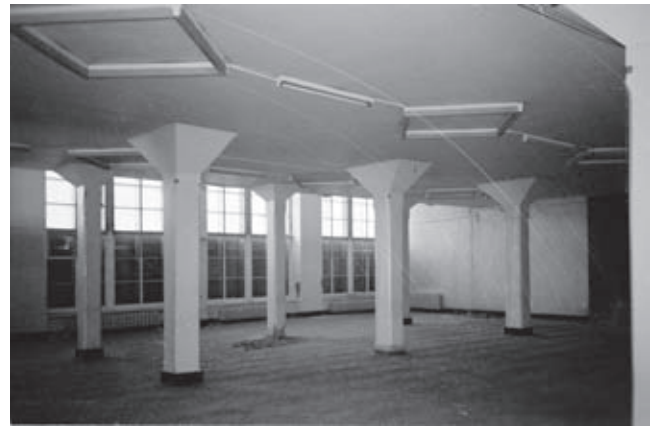
Burevestnik workers club, Moscow, 1927–29, arch. K. Melnikov. Vestibule before the restoration in 2000
