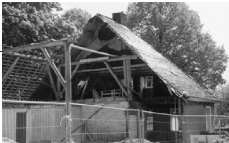
A farm in reconstruction, showing the traditional structure. Will the result of this building activity meet the standards of the Venice Charter?
