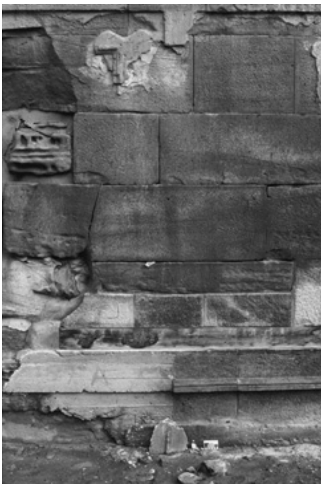
Qasr al Bint, condition of stucco decoration
