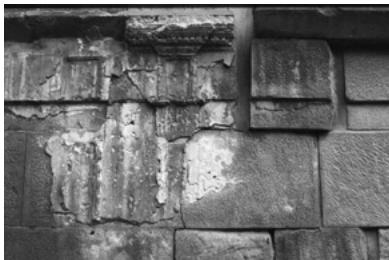
Qasr al Bint, recent rupture on stucco decoration
