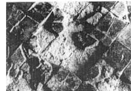
Fig. 4 - Indents of missing tiles on mortar bed, after treatment.
