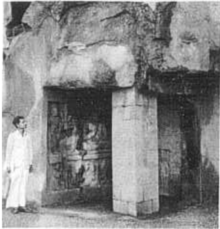
Pl. 4 - Ellora. Masonry pillar supporting the cracked roof of the cell in front of shrine 3.
