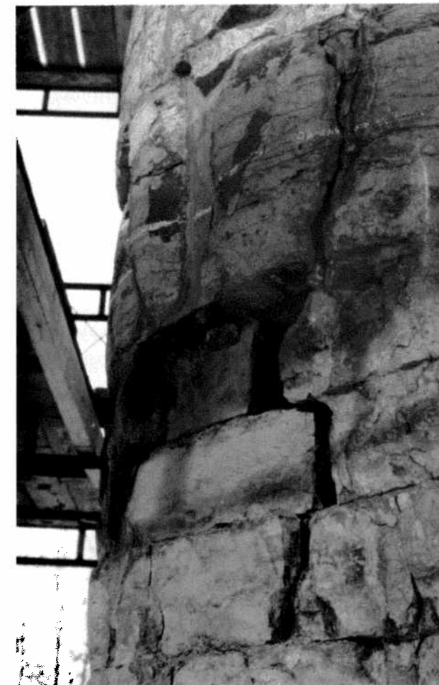
Frost damage on one of the pillars of the ruined cathedral at Hamar.
