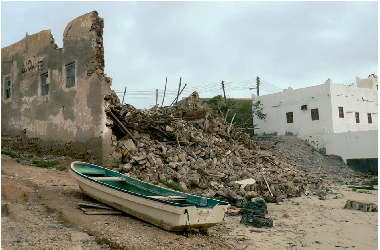
Mirbat, damage caused by a rain storm, 2007 (Photo: M.Pz.)
