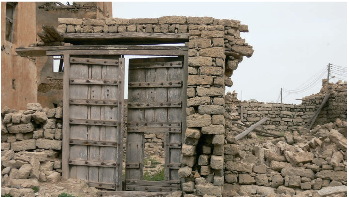
Mirbat, decaying entrance door (Photo: M.Pz.)
