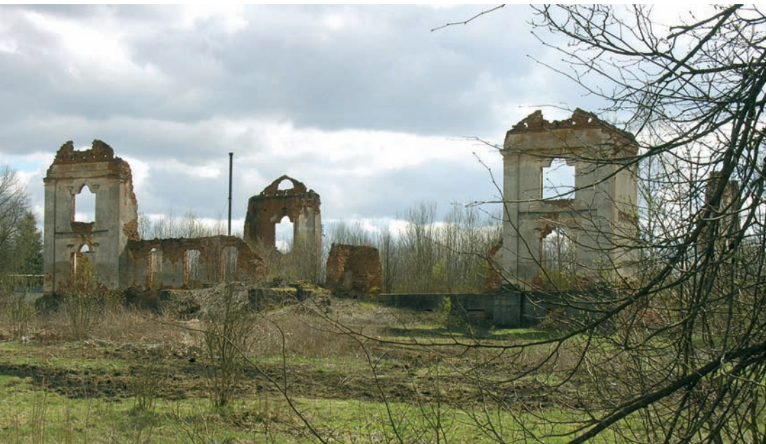
Remains of the famous Pavlovas' Merkinė manor estate in decay (Photo: Indrė Kačinskaitė Centre of Cultural Heritage, 2007)
