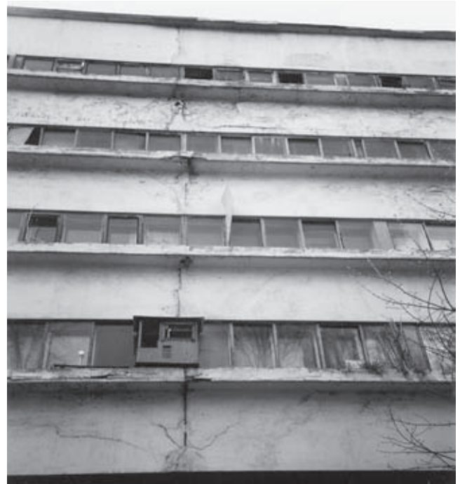
Narkomfin commune house of the Ministry of Finance on Novinsky Boulevard 25, Moscow, arch. M. Ginzburg, I. Milinis, 1928–30. East façade, 2004
