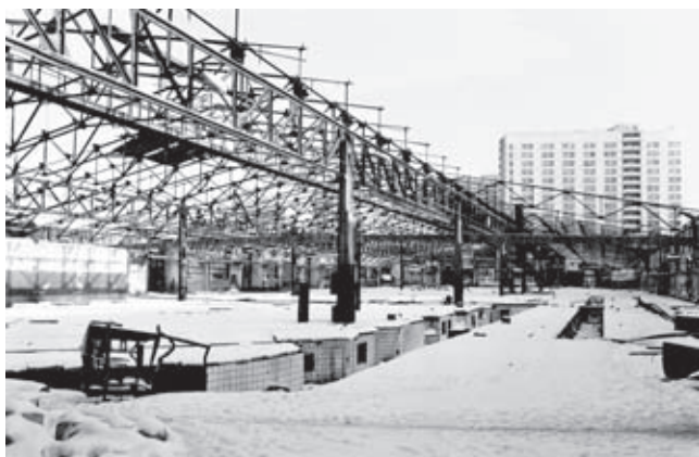
Bakhmet'jevsky-Park bus garage, Obraszova Street 19a, Moscow; arch. K. S. Melnikov, 1926–27, monument of local importance. The roof trusses were illegally removed in 2002
