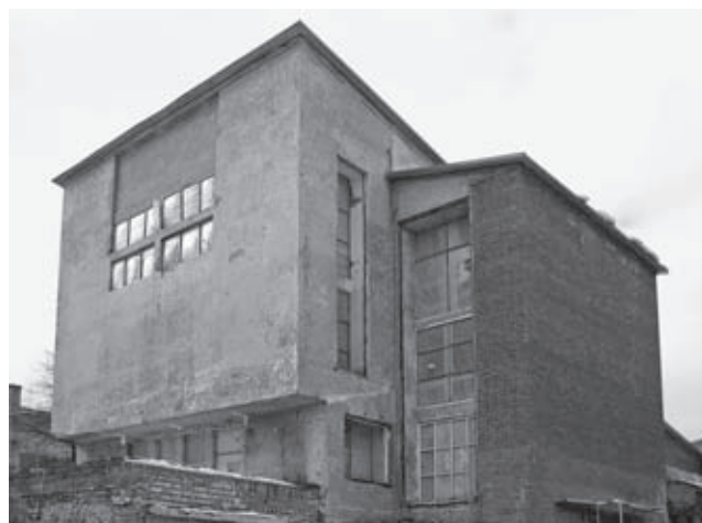
Frunse workers club of the "Dorchimzavod" chemical factory, Berezhkovskaya Naberezhnaya 28; Moscow, arch. K. S. Melnikov, 1927–29, monument of local importance. View in 2005, after a fire it was reconstructed
