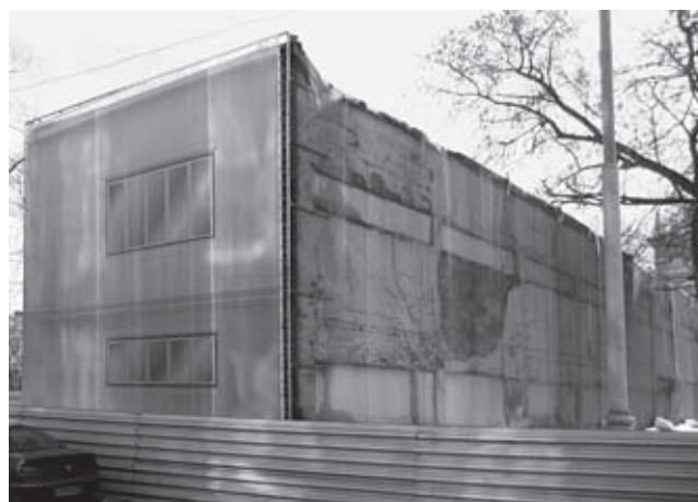
Laundry of the Narkomfin-House on Novinsky boulevard, Moscow; arch. M. J. Ginzburg, I. Milinis, 1928–30. Facade facing the Gardenring wrapped with fabric, 2006
