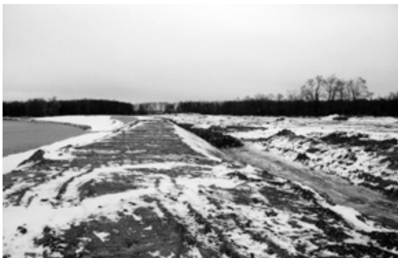
Veltrusy, a newly built dike on the western side of the park
