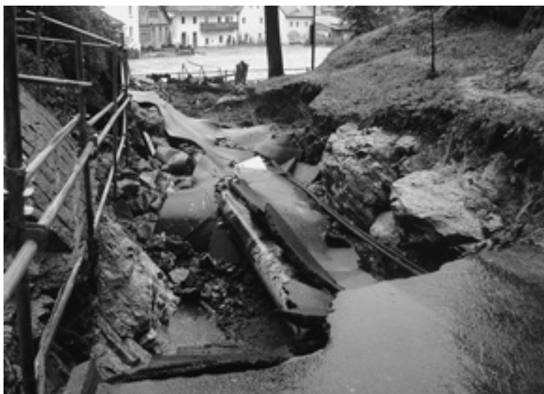
Český Krumlov, the condition of the access road under the Plášťový Bridge after the water falling off
