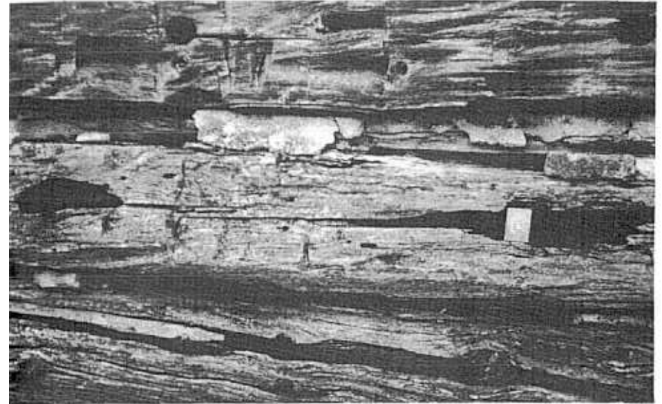
8. Heavy attack by carpenter ants ( Camponotus Pennsylvanicus ) in Eastern White Cedar logs in a nineteenth century log farm building, Ottawa, Ontario. Photo: Martin Weaver.
