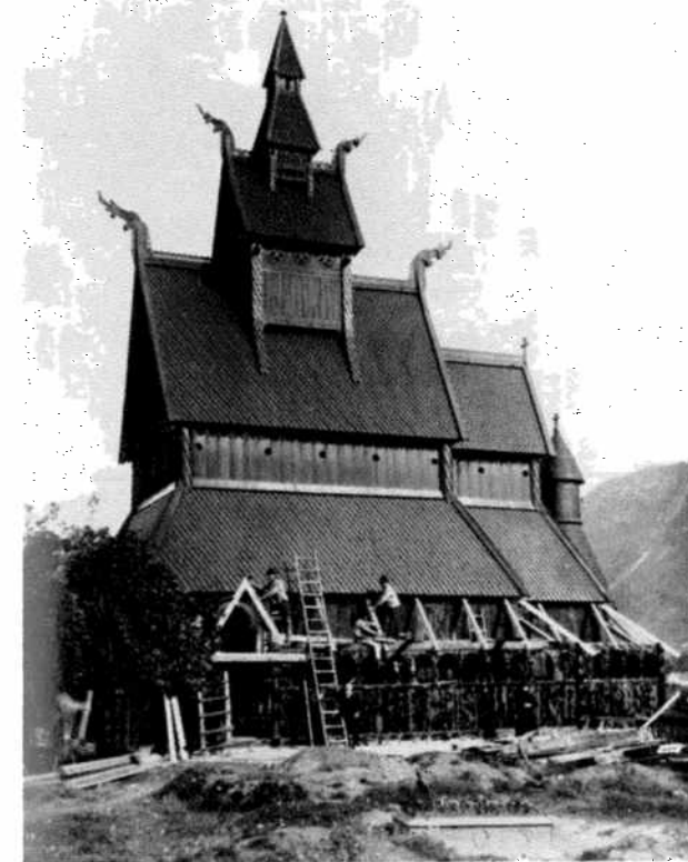
Hopperstad stave-church, Sogn & Fjordane, undergoing repair and restoration in 1889 (cf. preceding illustr.).
