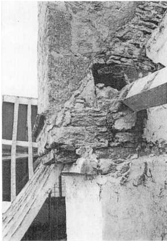
Fig. 16. — The condition of the base of the central chimney stack as revealed by opening-up.
