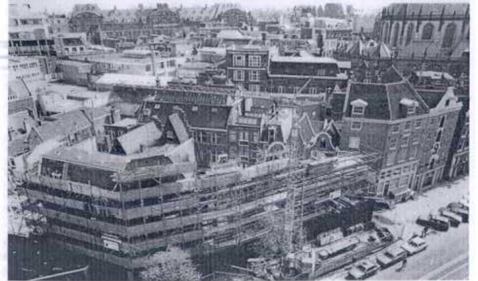
FIGS 13 and 14. The Blauw Erf project, the largest undertaken by StadsHerstel. In the upper photograph work is in progress on the first phase to the right, while the buildings on the left of this view show the seriously dilapidated condition of all in the group. The lower photograph shows the first phase after completion, and work in progress on the other buildings.
