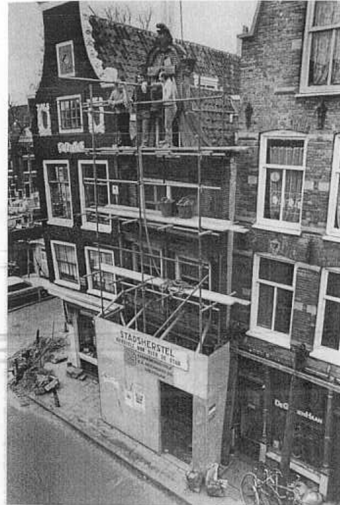
FIG. 18. 38 Herenstraat. This very dilapidated, heavily shored-up building was restored in less than one year. Completed in 1980, it is now an extremely desirable house and the ground floor shop is used by a dealer in old musical instruments. The facade was rebuilt, but the original gable decoration was re-used.
