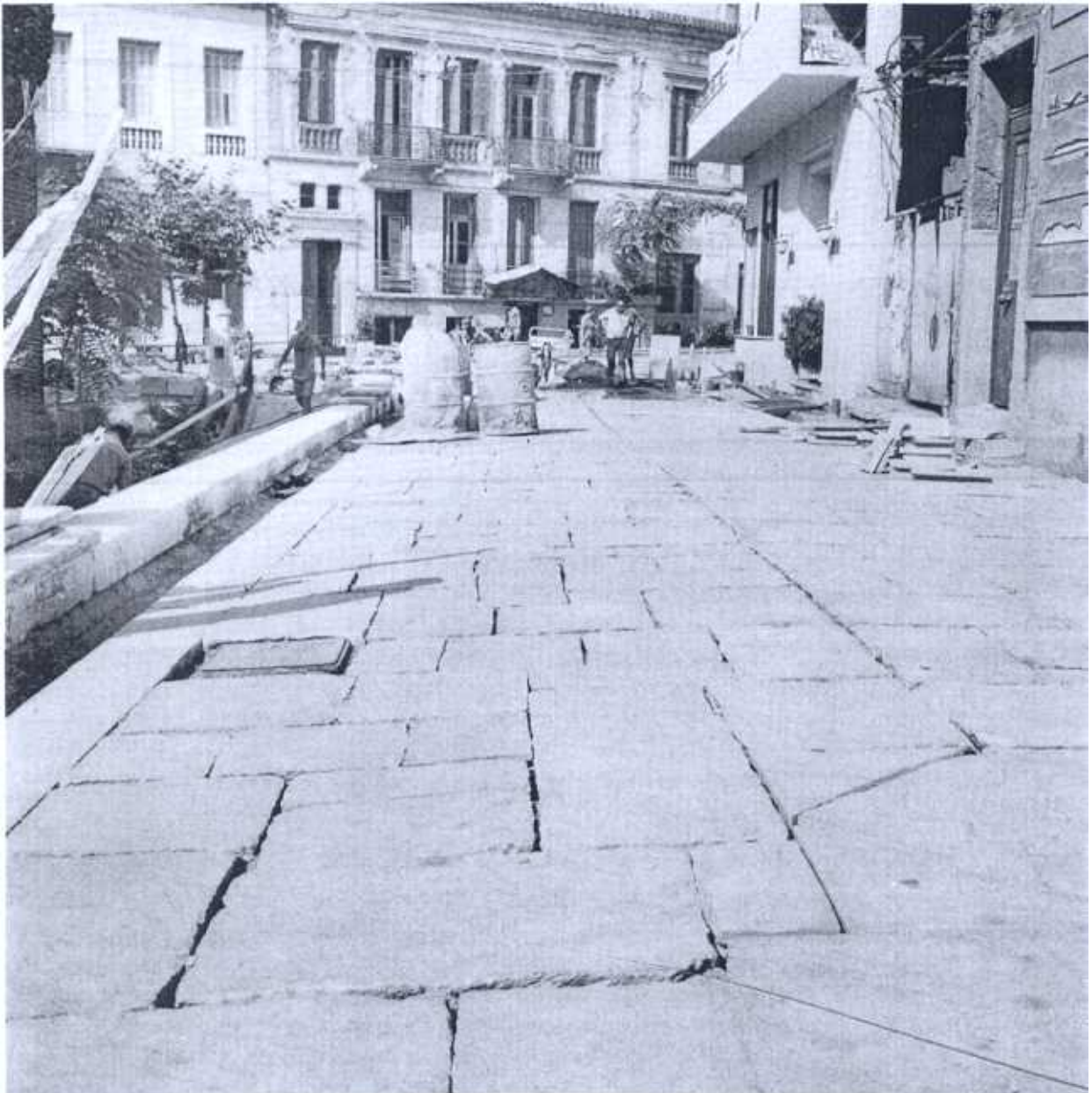
FIG. 1. The construction of the new pavements in the pedestrian area around Saint Katherine's Square.
