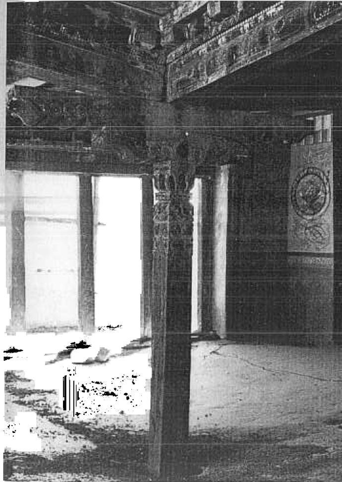
FIG. 15. The collapse of part of the south-eastern structure due to the removal of a pillar at level 4. At level 5 the pillar has literally punched through the floor, but at level 3 the structure has re-established itself. (Photo by John Sanday.)
