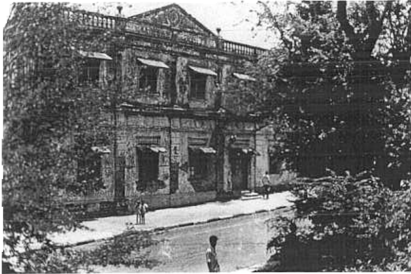
FIG. 11. A decaying building in Mihindu Mawatha, dating from the late nineteenth century.
