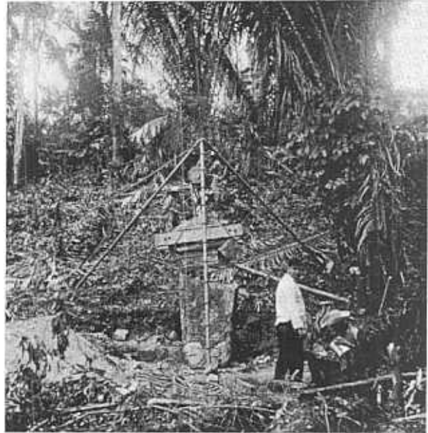
Fig. 21. — Placing the upper half of Stela 17 after setting the lower half in concrete in its altar platform.
