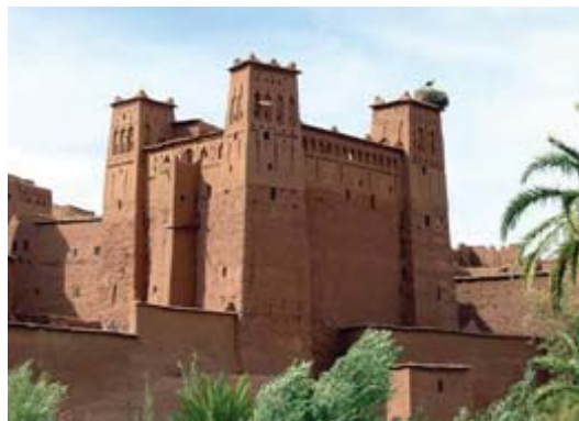
One of the hundreds of casbah in Morocco that are threatened by earthquakes and are in need of effective conservation strategies
