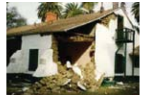
Recent shake-table research supported by the GCI have deepened understanding of how historic adobe structures perform in earthquakes
