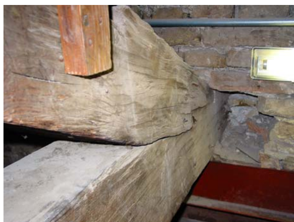
Figure 4. Joints details. Conjunction between the knee rafters and the tie beam. (N. Lombardini, 2007)
