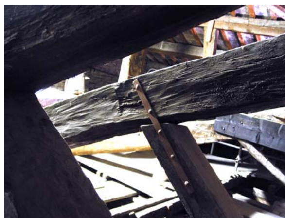
Figures 6,7. Examples of disjunctions between the struts and the knee rafter at several trusses (N. Lombardini, 2007)
