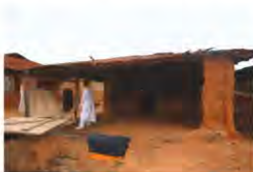
Photo 6. The exterior of the Obatala shrine in advanced degree of degradation.
