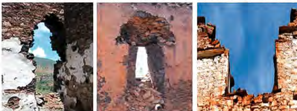
(Left) Collapse of stone wall above a lintel with formation of arch – Area01m at Level-1 (Middle) Collapse of stone wall above a lintel with formation of semi dome – Area01l at Level-1 (Right) Collapse of entire stone wall above a lintel – Area02c at Level-2
