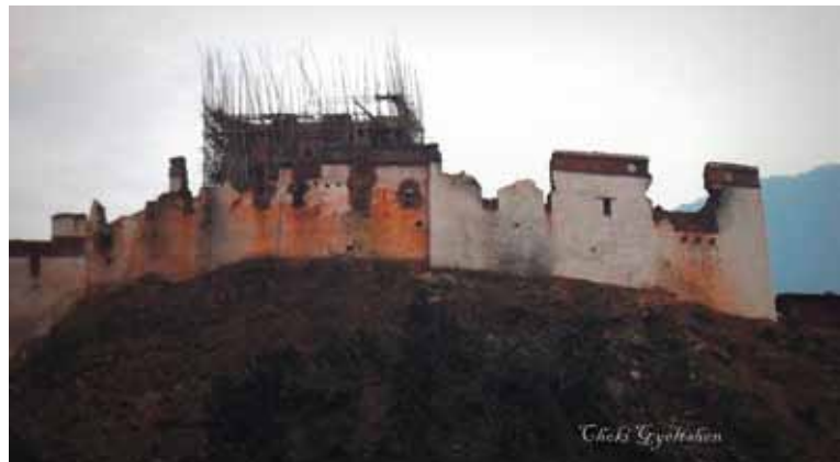
The ruins of Wangduephodrang Dzong after the fire (photos: Yeshey Dorji, Choki Gyeltshen)
